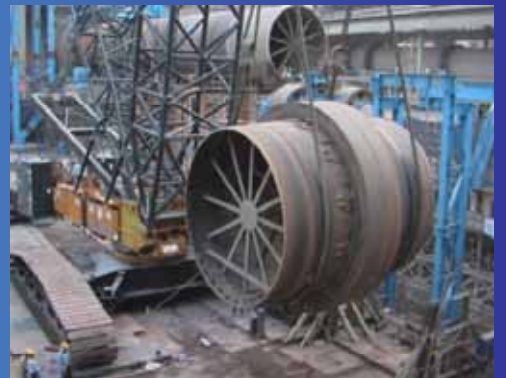
Installation for Kiln & Tire
