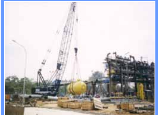
Installation for Slug Catcher
