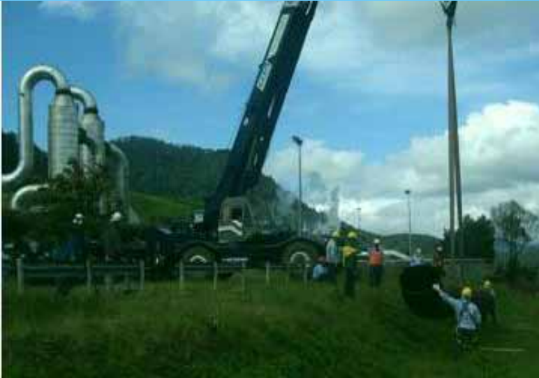
Pipe Line for Geothermal Power Plant
