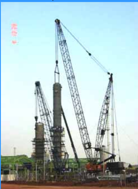
Installation for CO2 Absorber
