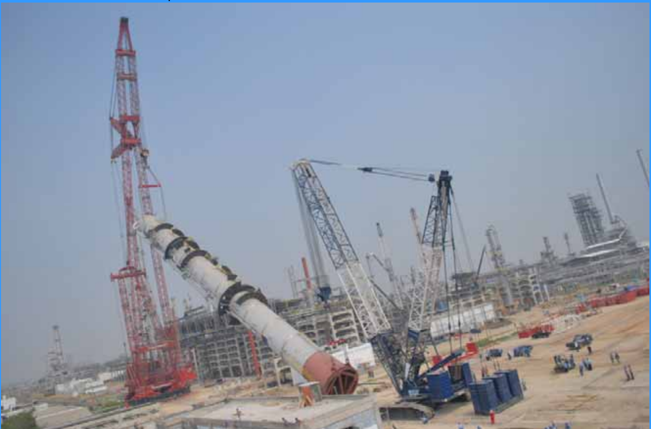
Installation for Deisobutanizer
