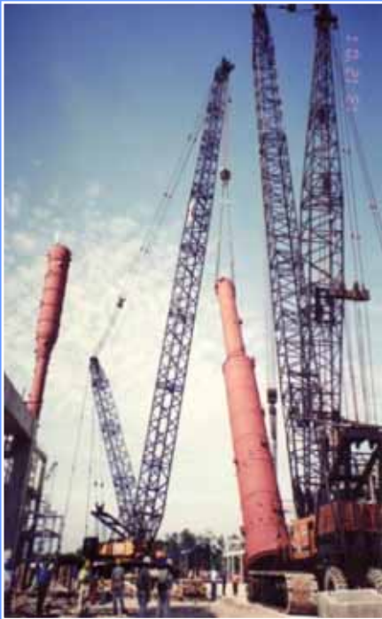
Installation for CO2 Absorber
