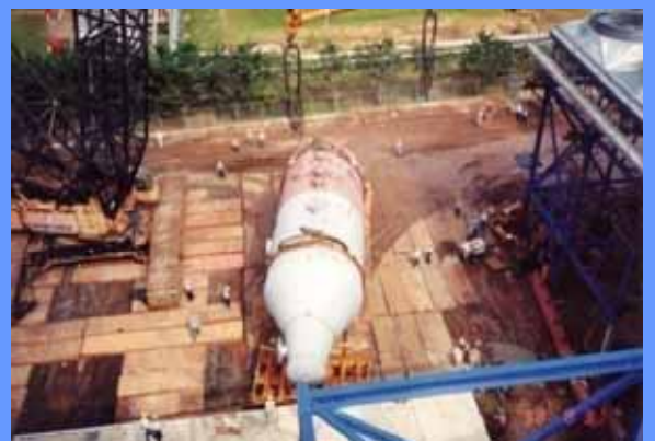
Transportation for Heat Exchanger
