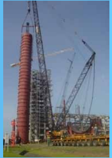
Installation for Deisohexanizer
