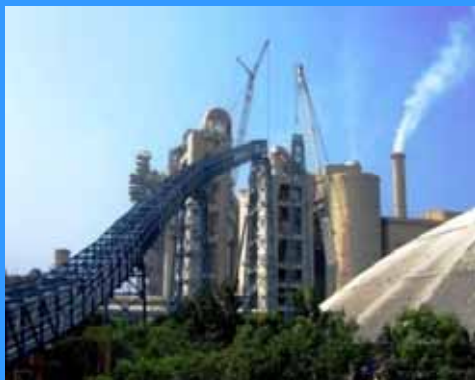
Installation for Conveyor
