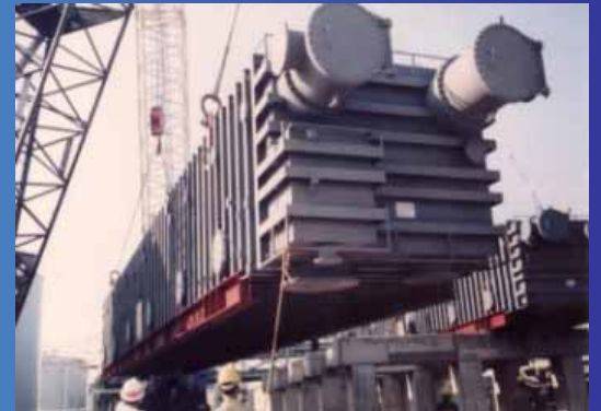
Installation for Desalination unit
