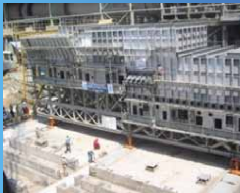
Assembly and Shifting Grate Cooler
