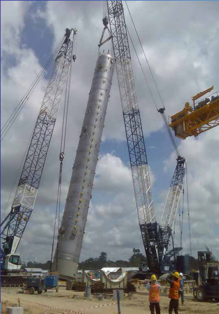
Installation for Absorption Tower
