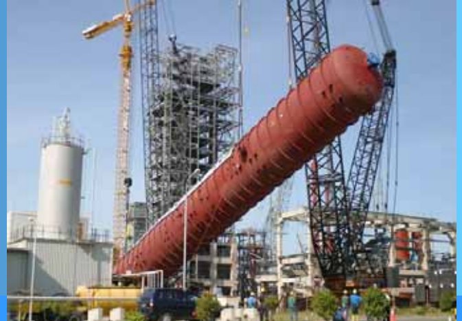
Installation for Deisohexanizer
