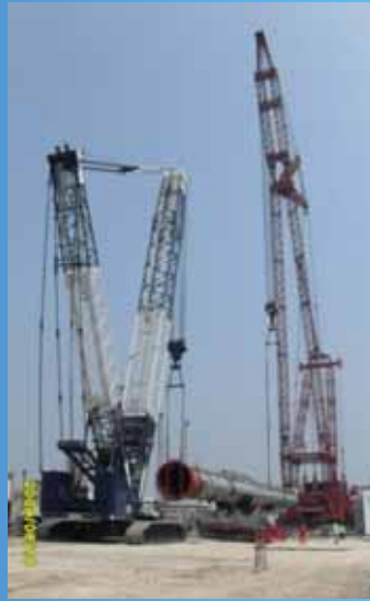
Installation for Deethylenizer
