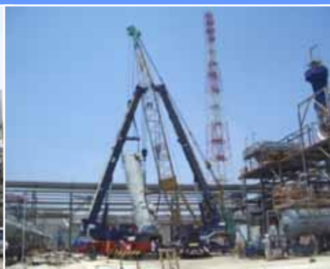
Installation for Amine Contactor
