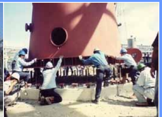
Installation for Reactor
