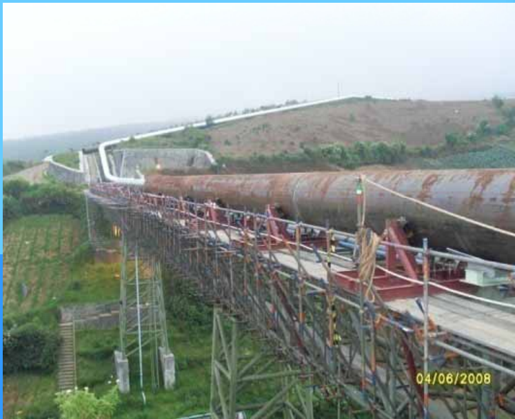
Pipe Line for Geothermal Power Plant
