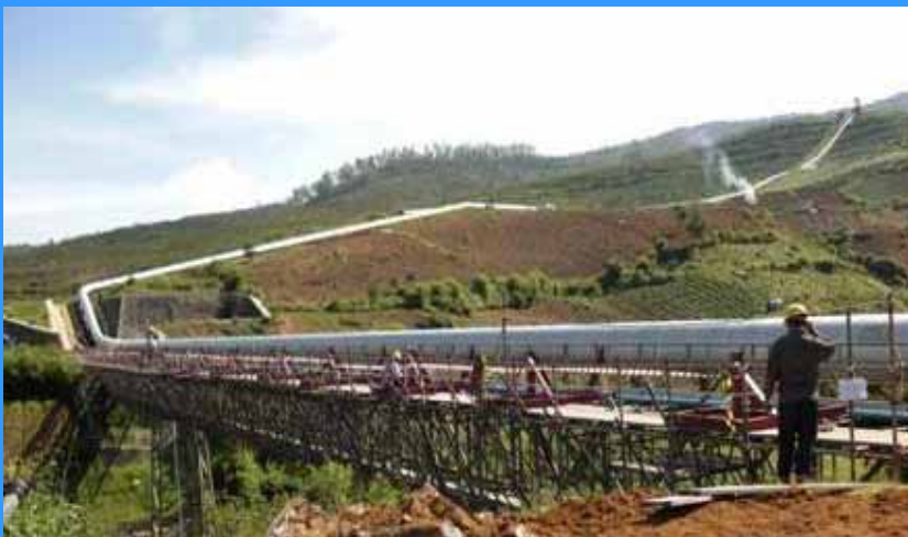
Pipe Line for Geothermal Power Plant
