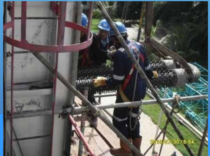
Re-tubing for Radiant Tubes
